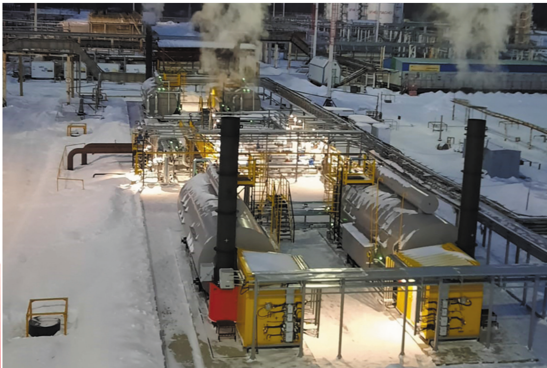
MUN Mobile Heating Unit
