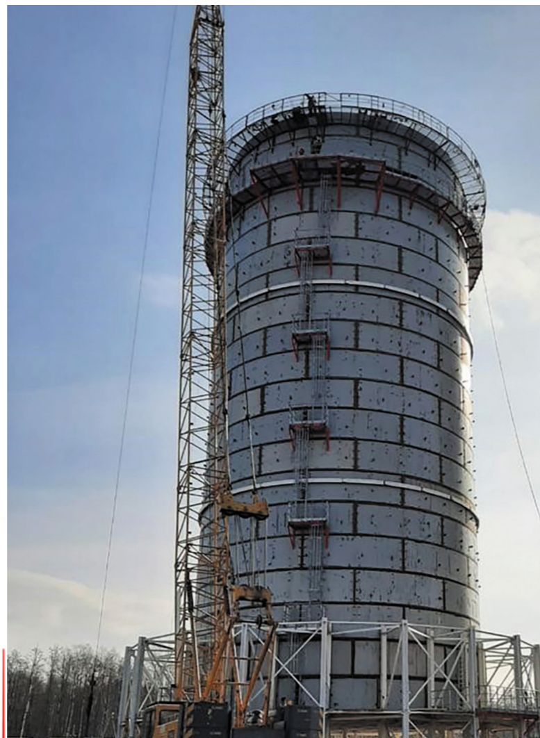
UFBG-ZT Enclosed type flare system after the installation of the metal structure
