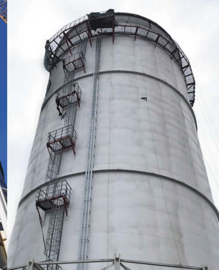
UFBG-ZT Enclosed type flare facility during installation
