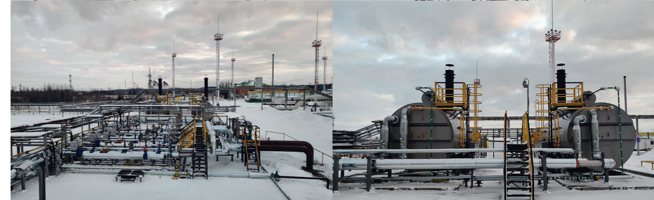
MUN Mobile Heating Unit
