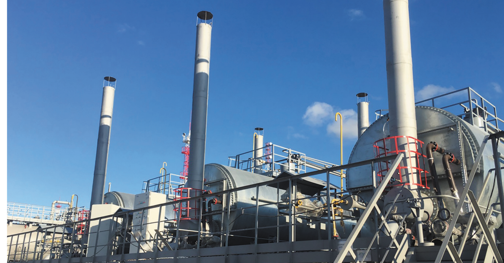
PP-1,6 heater at the client's facility
