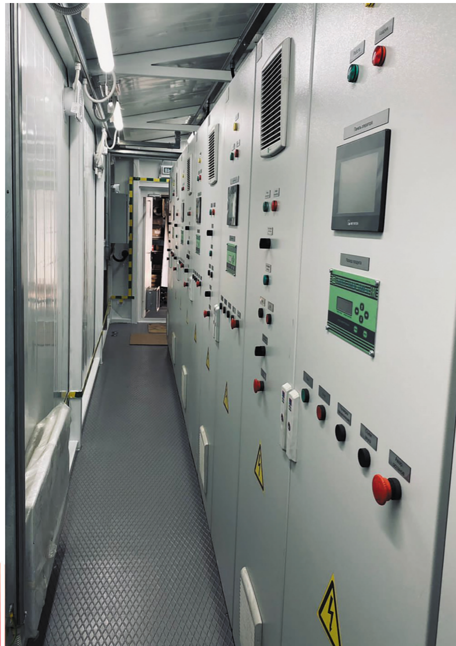
Automation system cabinets
